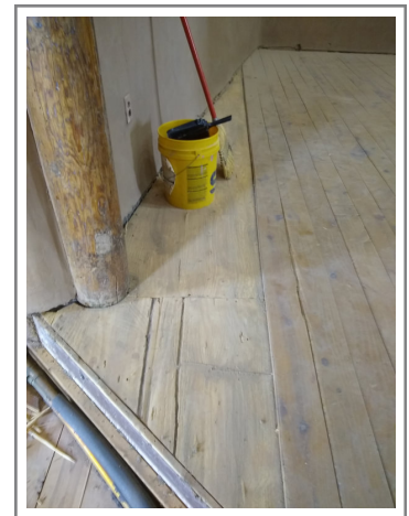
Severe cracks on the Old Church stage
